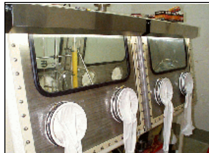
These gloveboxes are being modified to support larger Ac-225 shipments required by human clinical trials
